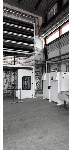
Onsite hydrogen production
