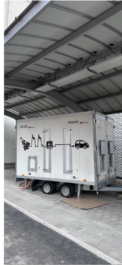
Battery buffer storage
